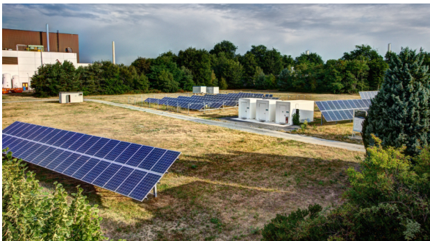
PV facility with Lithium-ion storage system
