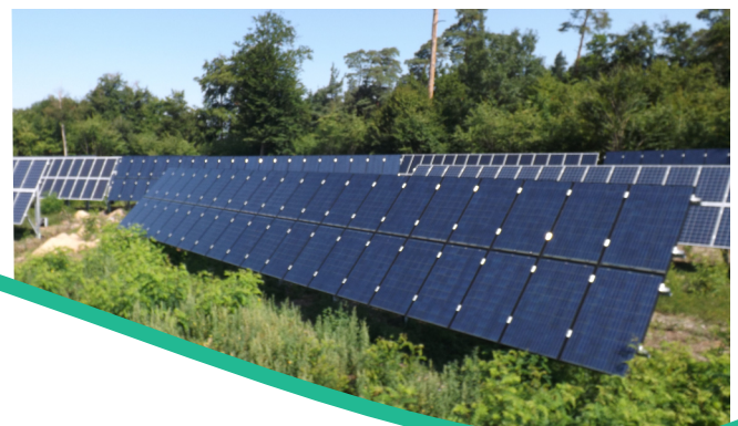
PV panels with different orientations
