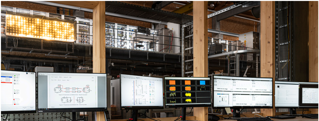
Control Room SESCL
