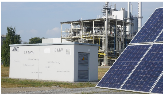
Compact lithium-ion storage system in the research environment at KIT
