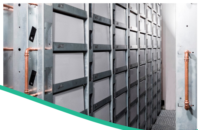
View into the battery room: Battery modules (white), shelving system, and copper cooling pipes.
